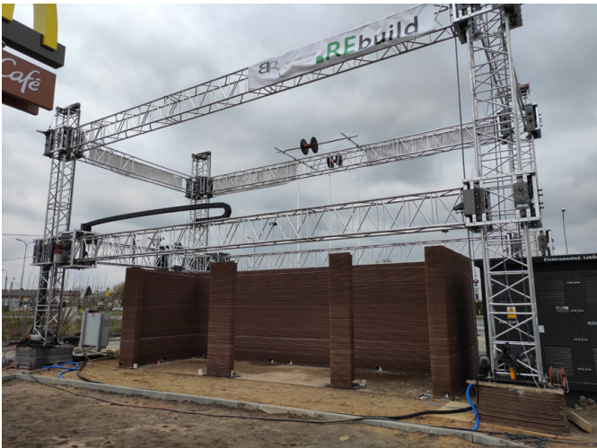
Fig. 2. Printer Rebuild v3. Real view from the first building site of this type in Poland, with the application of concrete in 3D printing
